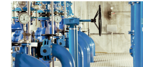
Supplying water for the City of Schwerin
